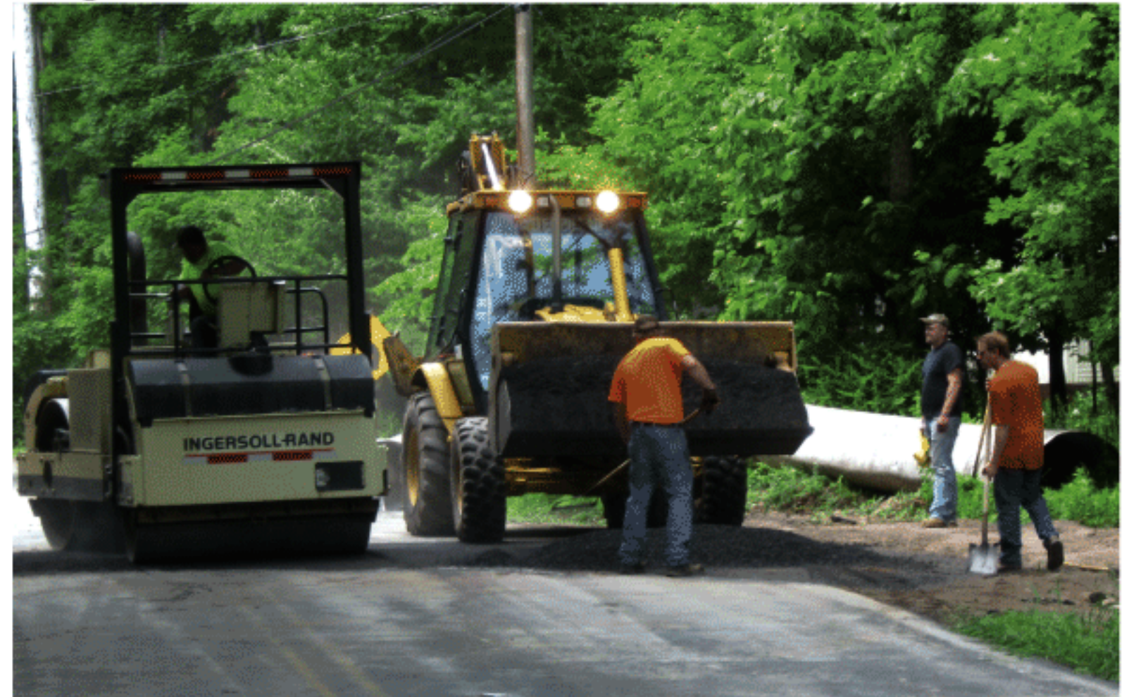
During the past few weeks, the Town of Denning Highway Department road crew was busy preparing heavily damaged areas along Peekamoose Road for black topping.
